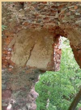
Ruins of the masonry
